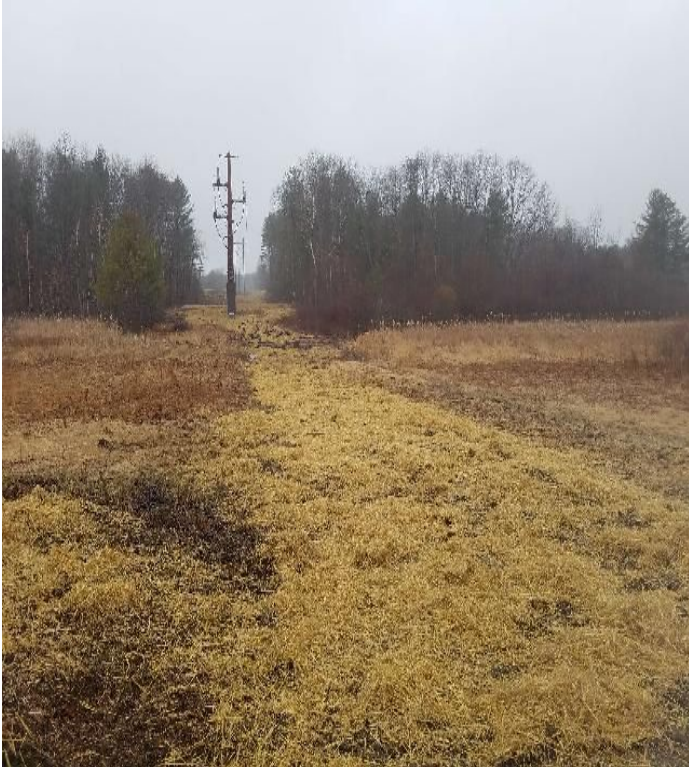
Fig 21: Crew seeded and mulched area after timber mats have been removed at Frink farm. Viewing west. (03-17-20).
