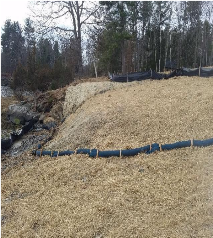
Fig 3: BMPs at toe of slope at Getchell property/west side of the Bay. Viewing south. (03-12-20).
