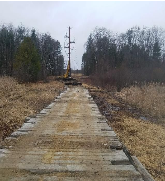
Fig 19: Beginning to remove timber mats at Frink farm and through Knights Brook. Viewing west. (03-17-20).
