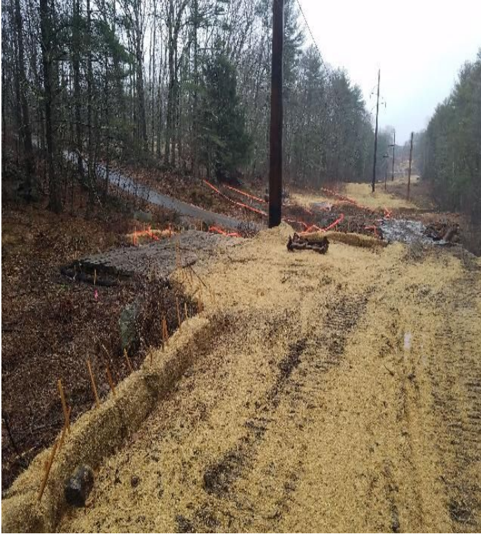
Fig 13: Exposed soils mulched with straw at Str. 63. Viewing west. (03-13-20).
