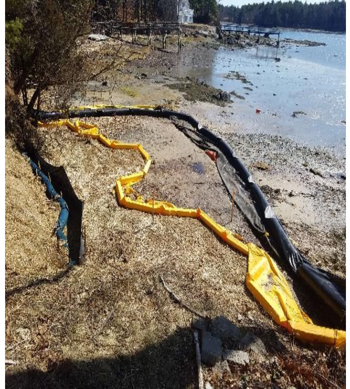
Fig 18: Turbidity barrier in intertidal zone at Gundalow landing/east side of the Bay. Viewing south. (03-16-20).
