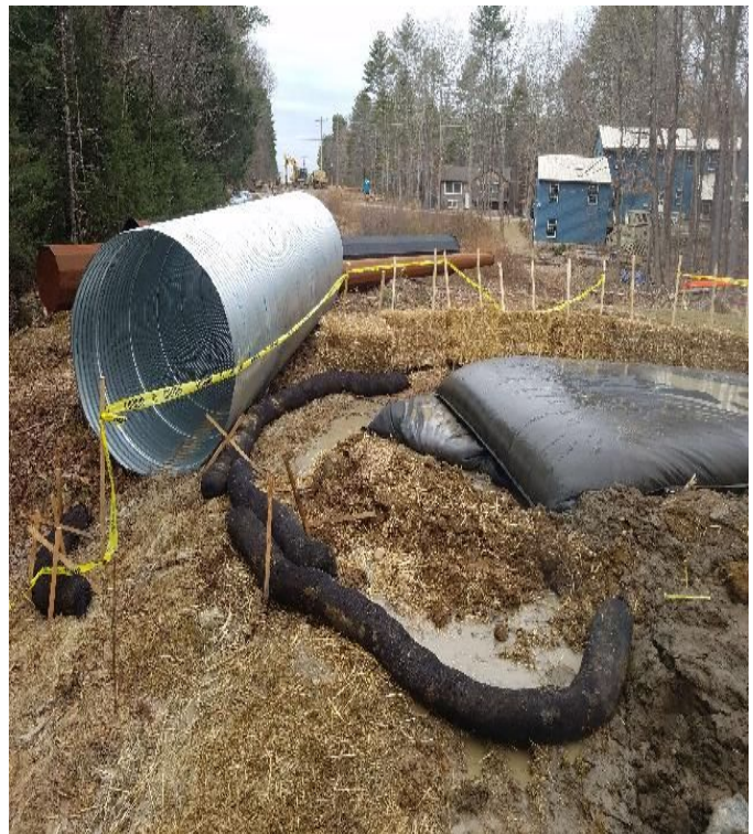
Fig 4: Using filter bag in upland area to dewater hole at Str.67. Viewing west. (03-12-20).
