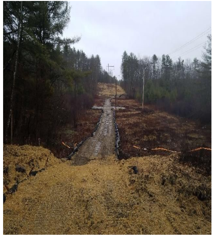
Fig 10: Access road through wetland DW31 and work pad for Str. 3162-13. Viewing east. (03-13-20).
